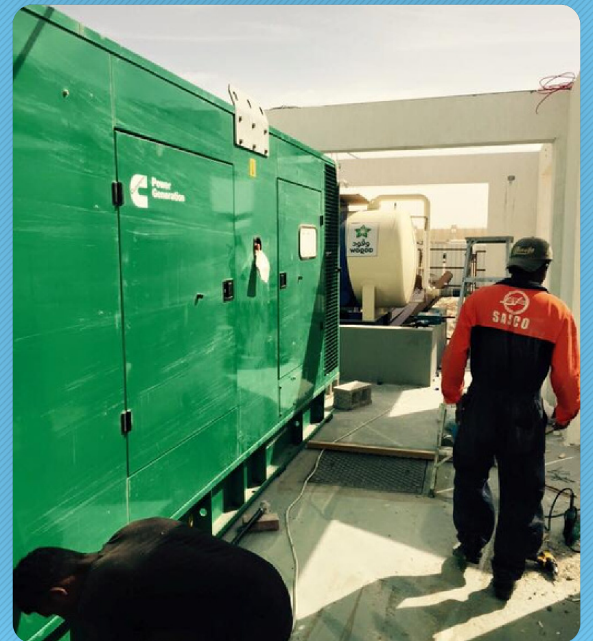
2000 KVA Generator & ATS Panel (Barazan Camp)
