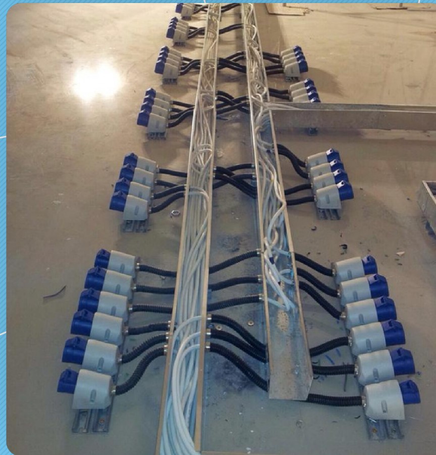
Data Center (Amiri Guard) Location: Barazan Camp - 2017
