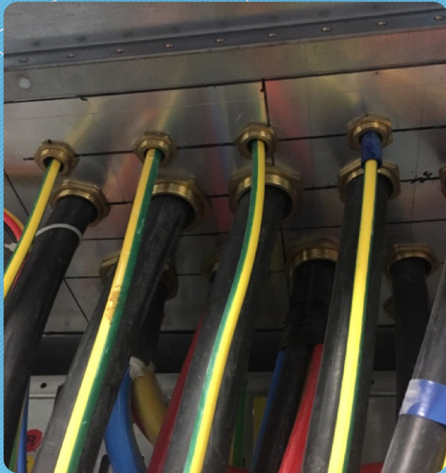
2500Amp MV Panels & Substations Many Different Location
