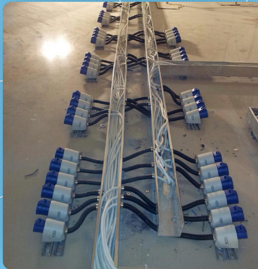
Data Center (Amiri Guard) Location: Barazan Camp - 2017
