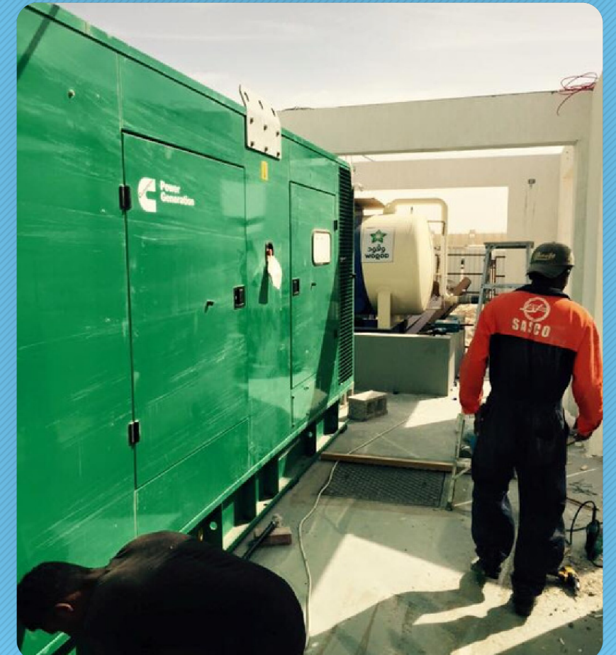
2000 KVA Generator & ATS Panel (Barazan Camp)
